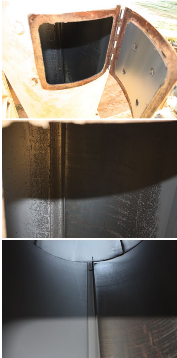
Figure 15. Angle-iron welded to the inside surface of cyclone cone at gin F.
